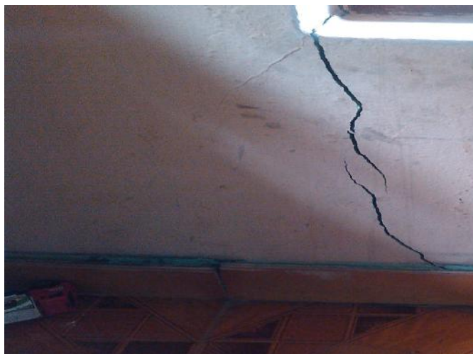
Fig. 1.11.1 Crack developed on the wall of a house at Vaniyamkulam
