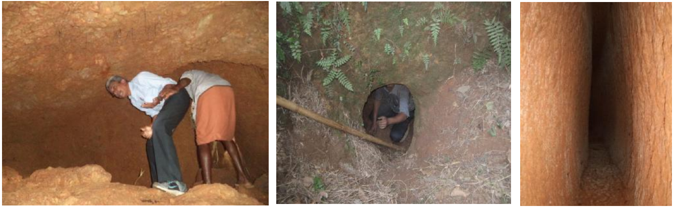
Fig. 1.10.3 Newly identified pipe and piping affected horizontal well Surangam (Tunnel) at Kuttikol in Kasaragod. Inside of the pipe (left), opening of the pipe (middle), Surangam / Tunnel (right)
