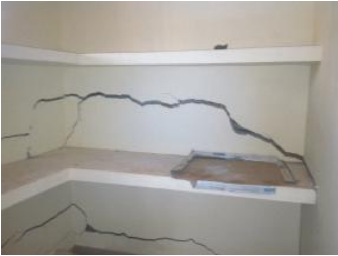
Fig. 1.13.1 Ground subsidence in Perumanna village, Malappuram dist.
