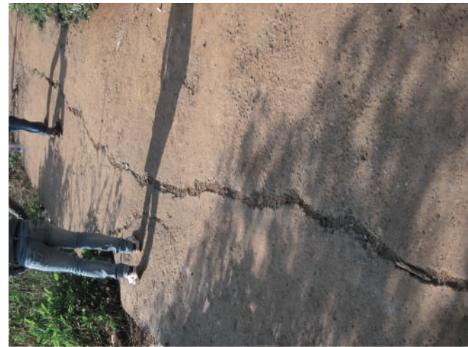
Fig. 1.11.7 Circular cracks have developed with creep damage in buildings and cemented road, Bhekavali Village, Mahabaleswar, Satara, Maharashtra
