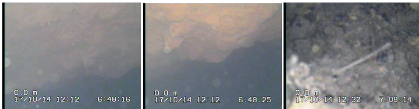
Fig. 1.10.10 The images taken by Push Camera from inside the pipes (filled with water)
