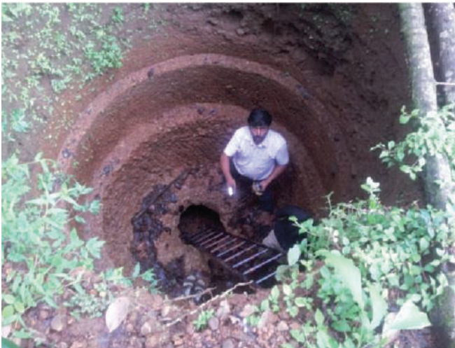
Fig. 1.10.2 Failed roof of tunnel inside the well, Niranganpara, Iritty taluk, Kannur district
