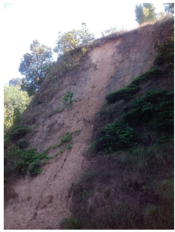
Fig. 1.11.2 Road section near Medikeri shows the presence of a crack in steep road cutting that can develop as a potential surface of failure
