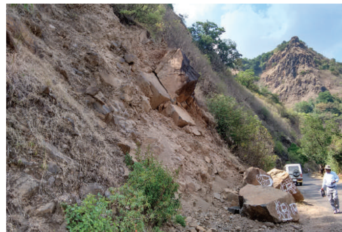
Fig. 1.11.4 Failed surfaces are the steep slopes of road cuttings with little vegetation cover.
