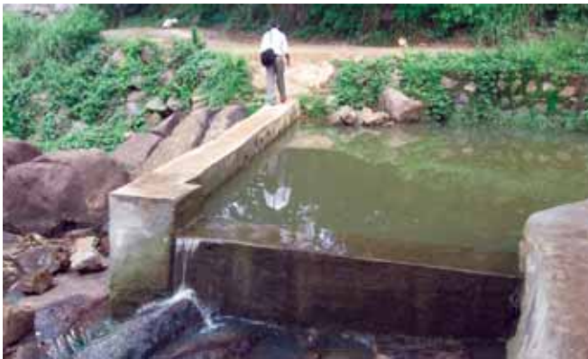
Fig. 3.1.1.1 Checkdam constructed in Mangad watershed of Chadayamangalam block arresting the surface flow and maintaining elevated water table conditions in the vicinity
