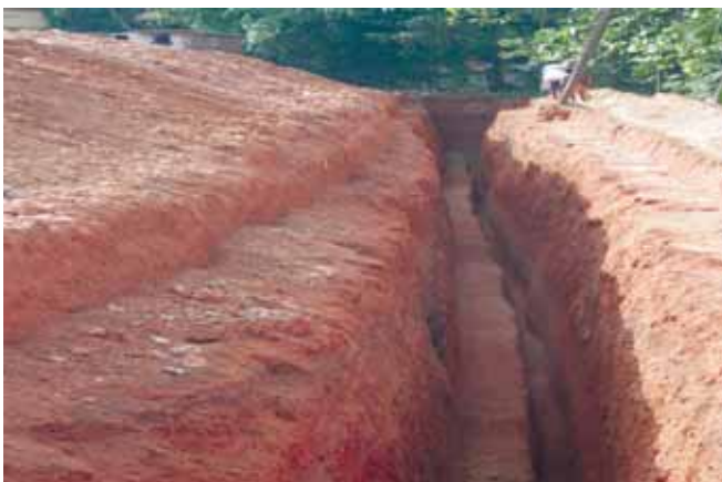
Fig. 3.1.1.2 The trench taken in laterite exposing the white clay layer. This trench is taken to provide a sub-surface dyke that maintains elevated water table conditions by preventing seepage of groundwater
