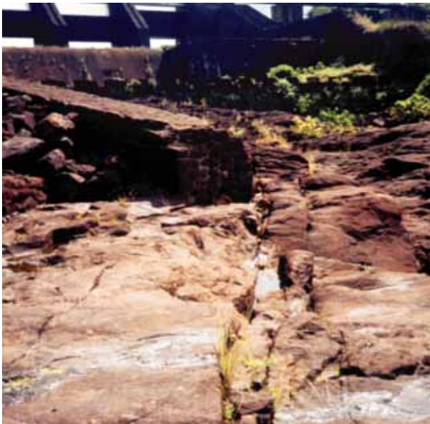
2.4.2.1 Closely spaced well-developed WNW-ESE oriented fractures are seen extending into the spillway section. These zones of weakness often display perceptible displacement of adjacent rock units
