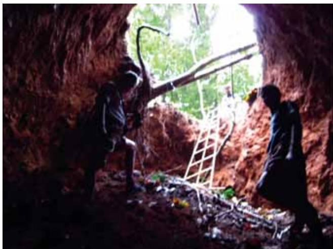
Fig. 2.1.1.2 Land subsidence due to soil piping at Udayagiri, Idukki on 14 th August 2010
